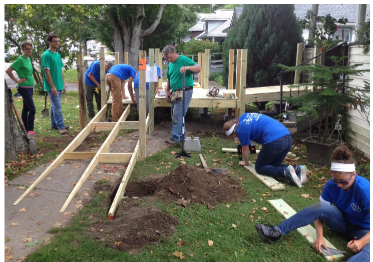
Broome County Council of Church's Ramp It Up program constructs a wheelchair ramp outside of a Broome County residence.
